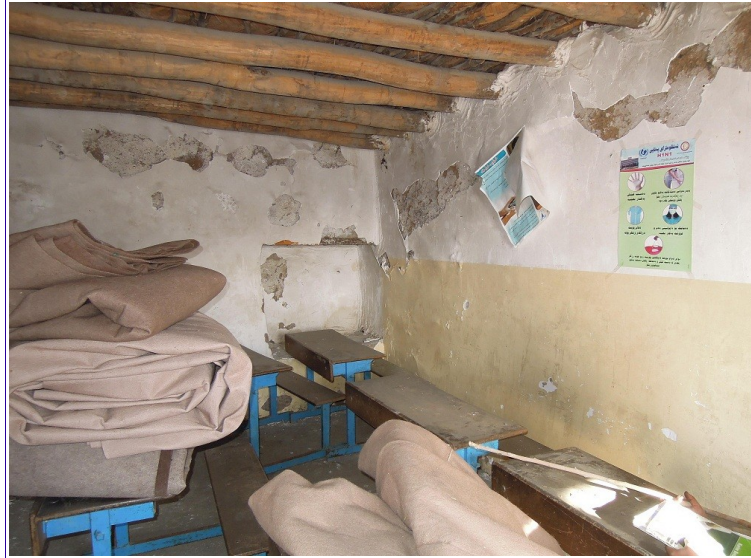
Shock wave damages to the school Zewgah village
